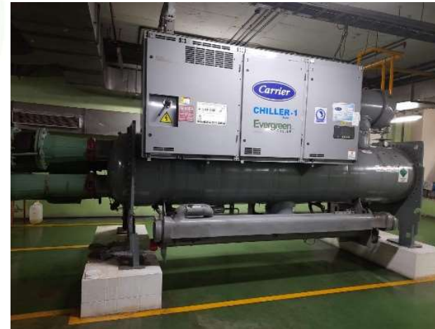
Energy Efficient Air Conditioning / Chillers
