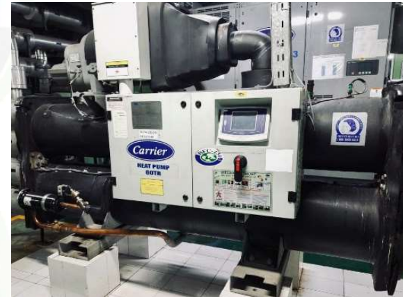
Heat Pump (Utilization of Waste Heat)
